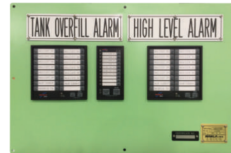
HIGH AND OVERFILL ALARM PANEL
